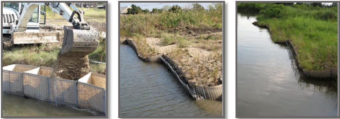
Figure 11. Hesco Delta Unit – A type of shoreline gabion system
